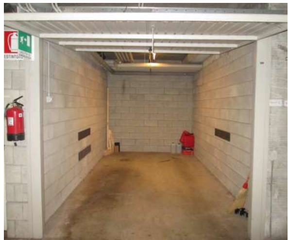
Locale box sub. 1091
