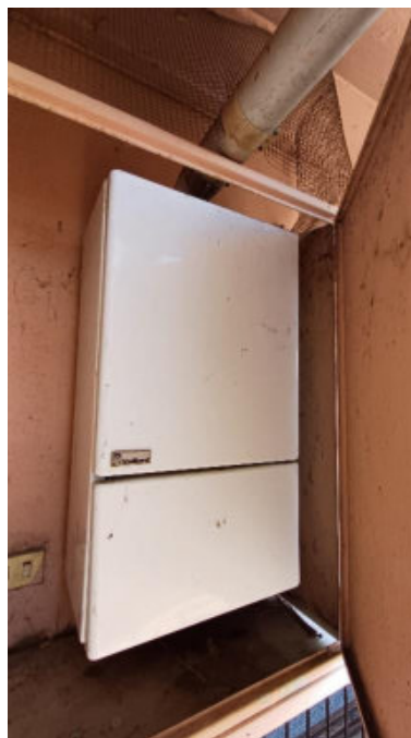
Caldaia a gas
